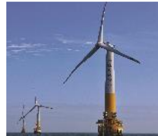
Putian Pinghai Bay offshore wind power
